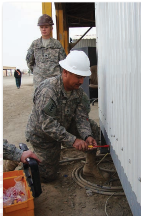
Staff Sgt. Jeffery Arth works to connect power to a trailer as Spc. Brianna Thompson waits patiently. Both Soldiers are deployed to Kuwait with the 188th Engineer Company (Vertical).
