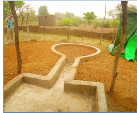
Latest Soak Pit Design: With concrete curb and private washing area (note: all soak pits may not represent this level of effluent containment)
