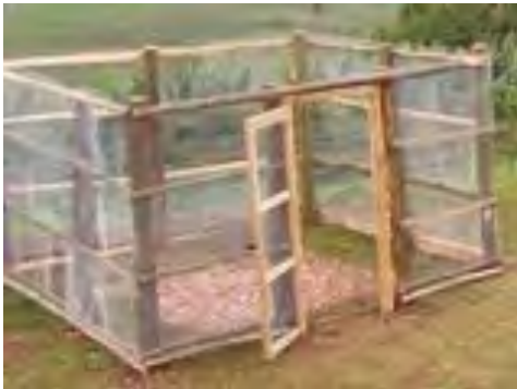
4: Soak pit area should be fenced to keep out children and animals
