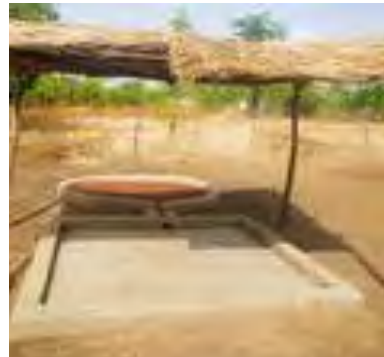
5: Soak pit area should be fenced to keep out children and animals
