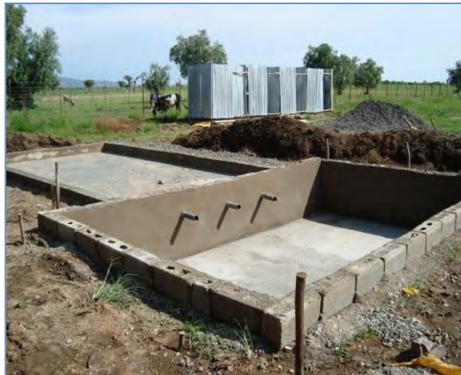
Evaporation Tank with wash area adjacent
