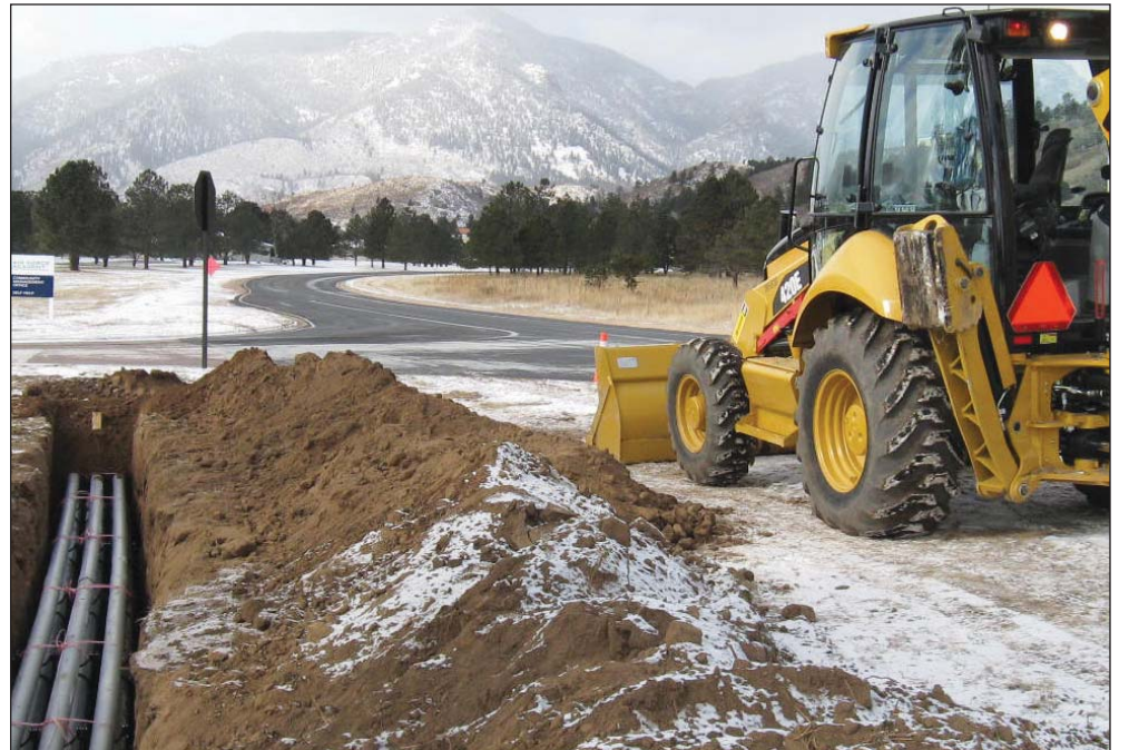
COURTESY PHOTO A CSU project outside of Pine Valley Housing shows what construction will look like this month when the Academy installs new gas and electrical systems in base housing.
