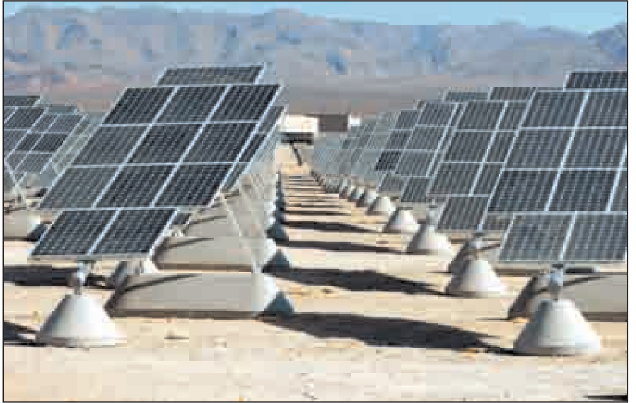
On 140 acres of unused Nellis land, 70,000 solar panels await activation as the first third of the solar photovoltaic array was commissioned Sunday. The other 66 percent of the panels will activate by late December.
