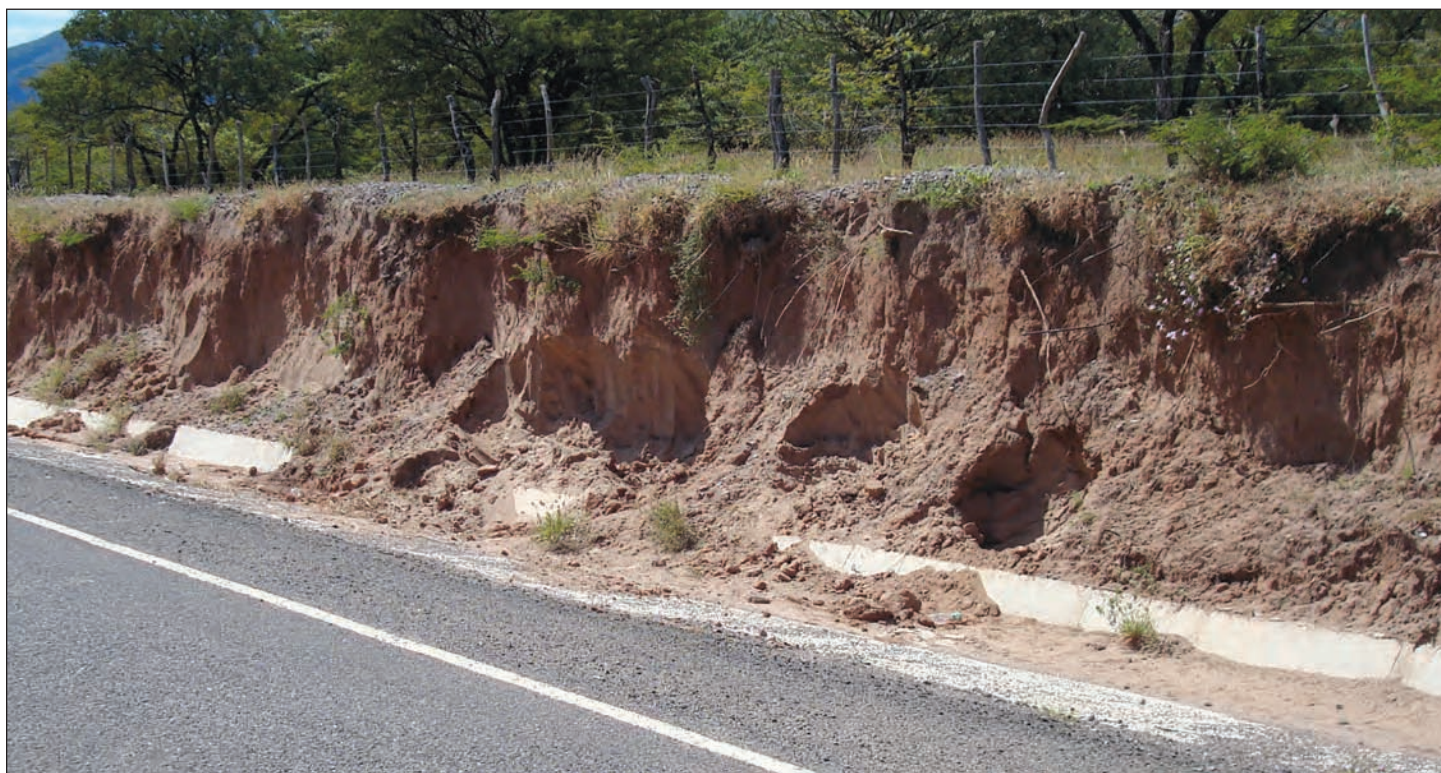
Figure 18: Erosion of Steep Slope along Secondary Road, Honduras Transportation Project
