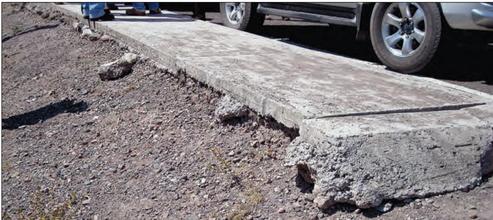
Secondary road: Lack of revegetation of fill slope resulting in erosion of fill behind and under sidewalk
