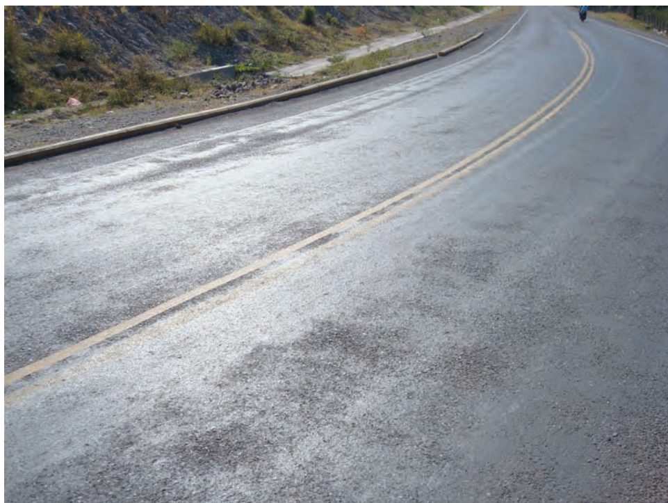
Figure 16: Flushed Asphalt on Secondary Roads, Honduras Transportation Project
