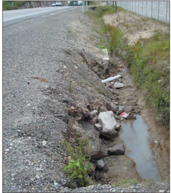
CA-5 Section 4: Lack of revegetation along edge of drainage ditch resulting in erosion
