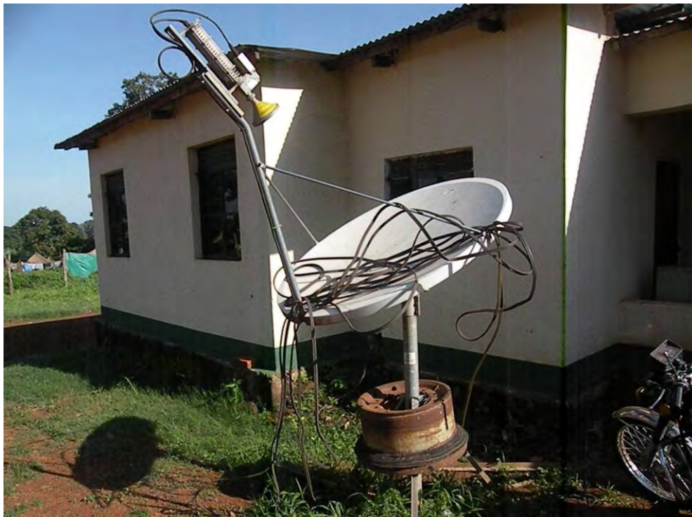
Old VSAT dish sits idle outside the Western Equatoria Ministry of Physical Infrastructure in Yambio. Sustainability of new VSAT system is critical
