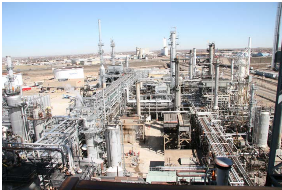
Figure 38. Overview of the Inside the SUNCOR oil refinery in Commerce City, CO.
