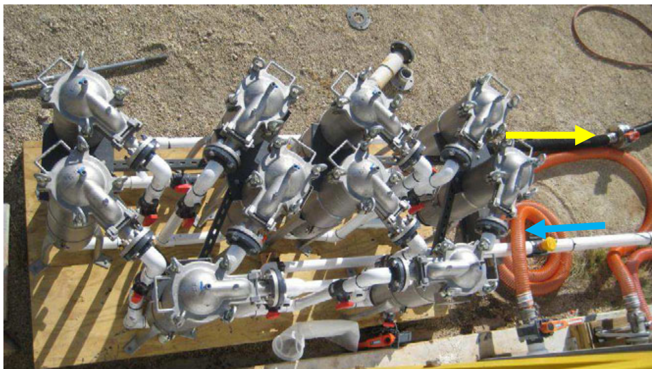
Figure 9. Plan view of the prototype filter skid at NRLKW. Blue arrow shows water entering the filter skid; yellow arrow shows water exiting the skid.
