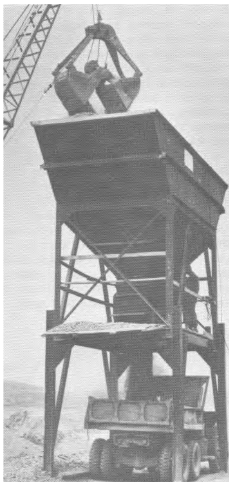
This truck is being loaded with a mixed crushed rock compound used in runway construction.
