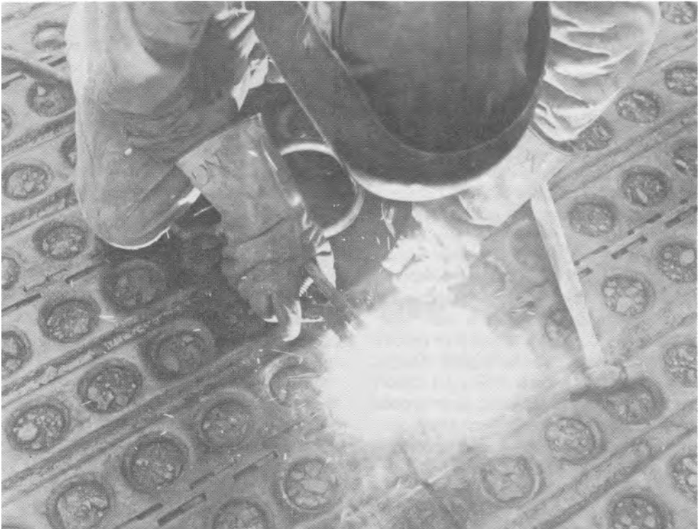
Locking slots and bayonet hooks are secured and welded by crews of the 930th Engineer Aviation Group of the U.S. Army.
