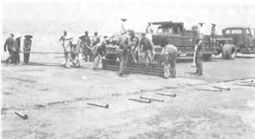
Upgrading the airfield at Tan Son Nhut, an Air Force construction team replaces pierced steel planking with new N9-M1 aluminum matting, August 1965.
