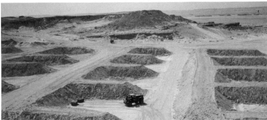
RED HORSE engineers tackled large and heavy jobs such as the creation of this munitions storage site.
