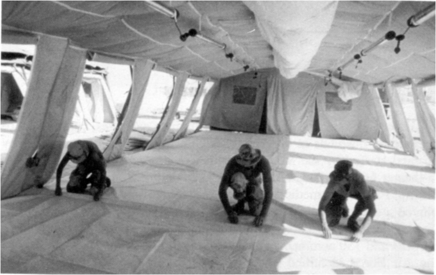
The backbone of the deployable medical treatment system is the air-transportable hospital, here being assembled by crews.
