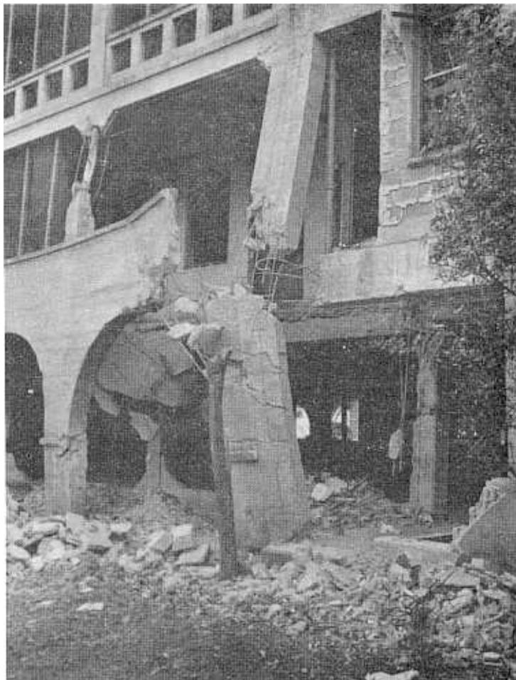
Badly damaged barracks of the 6th Pursuit Squadron, which suffered heavy casualties. (Joe K. Harding)
