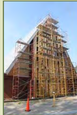
The newly renovated Turner facility will total 4,000 square feet and will be used for multiple activities on center.
