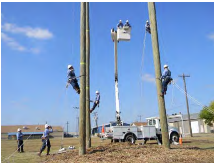
Students at the Gary Job Corps Center learn the importance of safety training and hands-on experience in their Overhead Line Construction classes.
