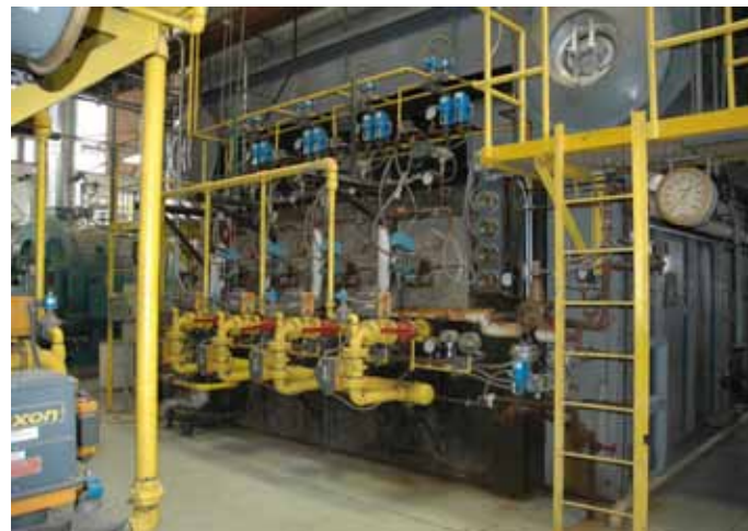
This is one of three central heat plants at Tinker AFB, Okla., that will be decentralized using an Energy Savings Performance Contract. The project could reduce natural gas consumption 40 percent and save up to $7 million. (U.S. Air Force photo/Bill Dalky)
