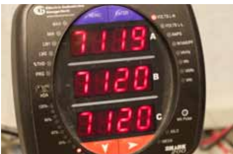
This electric meter is one of thousands across the Air Force that will soon be hooked to an advanced meter reading system. (U.S. Air Force photo/Eddie Green)
