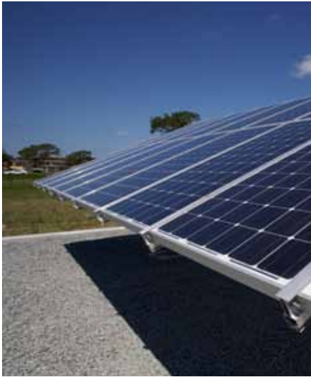
This solar array installed at AFCEC, Tyndall AFB, Fla., is just one of 212 renewable energy projects in operation on 89 installations. It is a small example of how the Air Force plans to meet goals in the One Gigawatt Renewable Energy Plan and the Net Zero Implementation Plan. (U.S. Air Force photo/Eddie Green)
