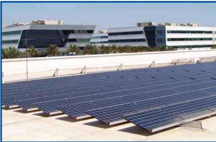
Photovoltaic Roof Project at Los Angeles AFB, California
