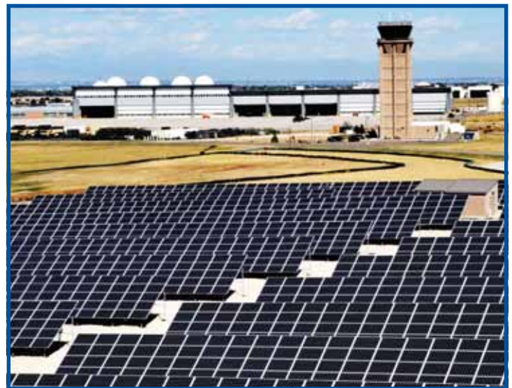
Photovoltaic Array at Buckley AFB, Colorado
