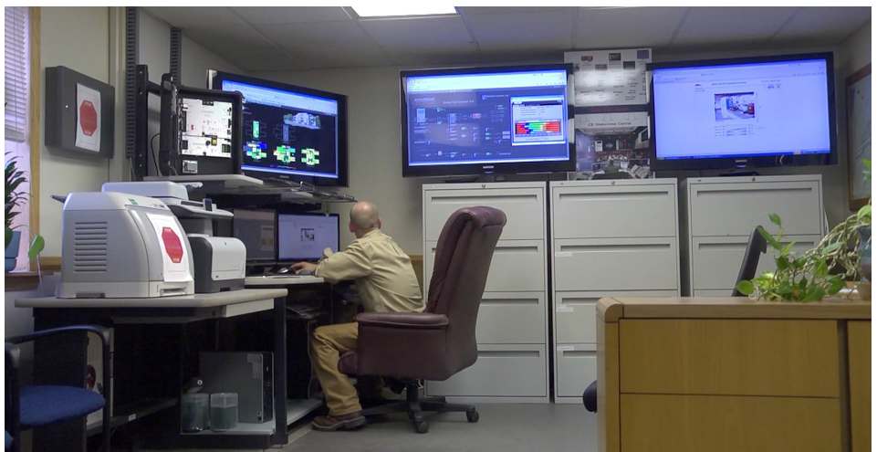
JBER, Alaska, uses a sophisticated energy management control system to monitor buildings and find energy savings. Currently the system saves the base over $500,000. (U.S. Air Force photos/Eddie Green)
