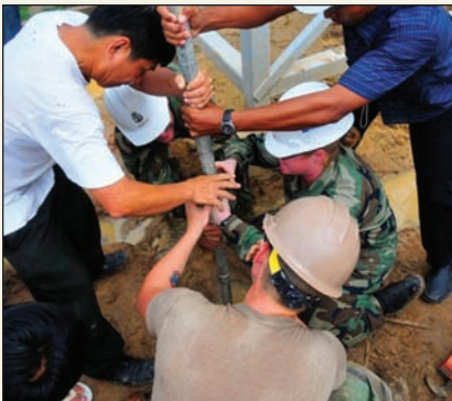
With the help of local Cambodians, Navy engineers work to complete a well-drilling humanitarian and civic assistance project as part of the Pacific Partnership 2010 exercise.
