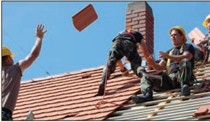
Hungarian and U.S. Army engineers work together to replace the roof of the Zalahalap Elementary School in the Hungarian village of Tapoica.
