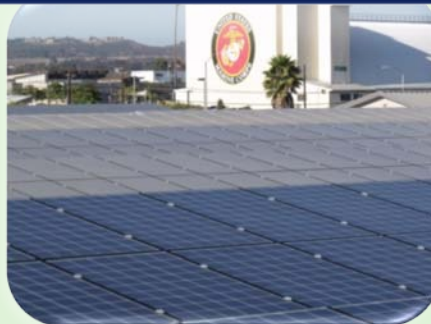
PV System MCAS Miramar
