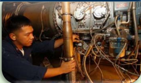
Allison 501k G/T Generator January 2011
