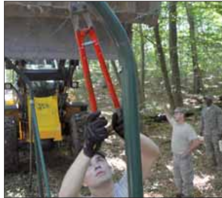
Rick Scavetta Airman 1st Class Michael Callaghan helps fellow 786th Civil Engineer Squadron Airmen remove fences from Kapaun Air Station, part of an effort to open up the area between Army and Air Force bases in Kaiserslautern.
