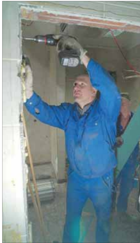
Shaun Maigitter, with the Army and Air Force Exchange Engineering Europe Team, removes part of a doorway at the Patrick Henry Village movie theater March 4. The three-man team is updating the concession area to provide better equipment for the employees to better serve their customers.
