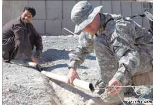
Spc. Christopher Kroneberger (right) helps an Afghan man lay cable at Forward Operating Base Lagman, Afghanistan, March 4.
