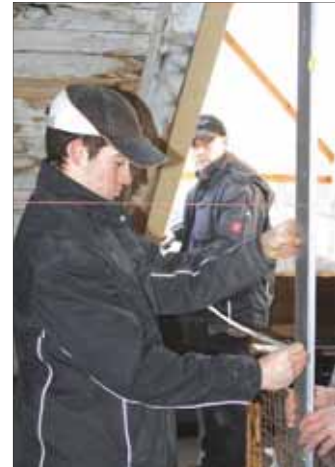
Mark Heeter Carpenters work on renovations to the future headquarters of the 7th Signal Brigade on Ledward Barracks in Schweinfurt.
