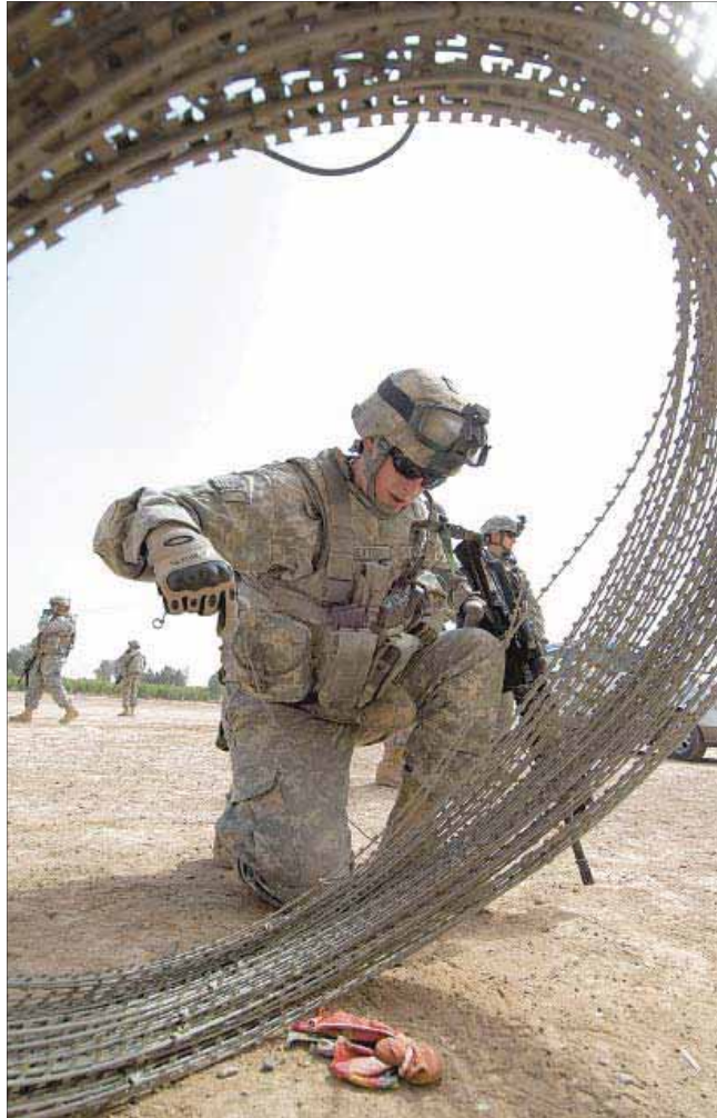
U.S. Navy Petty Officer 2nd Class Walter J. Pels Spc. Zachary Sexton deploys concertina wire around the entrance to a makeshift medical clinic in Abu Bakr, Iraq, April 7. Soldiers are preparing the facility for medical personnel from the Iraqi Ministry of Health, who will provide free medical care and consultation to area residents. Sexton is assigned to 1st Battalion, 24th Infantry Regiment, 1st Stryker Brigade Combat Team, 25th Infantry Division.
