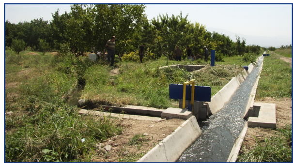
A tertiary irrigation canal in Armenia
