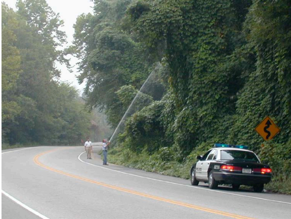
Fig. 17. Treatment of kudzu interfering with sight distance near intersection of Highway 95 and Bear Creek Road.
