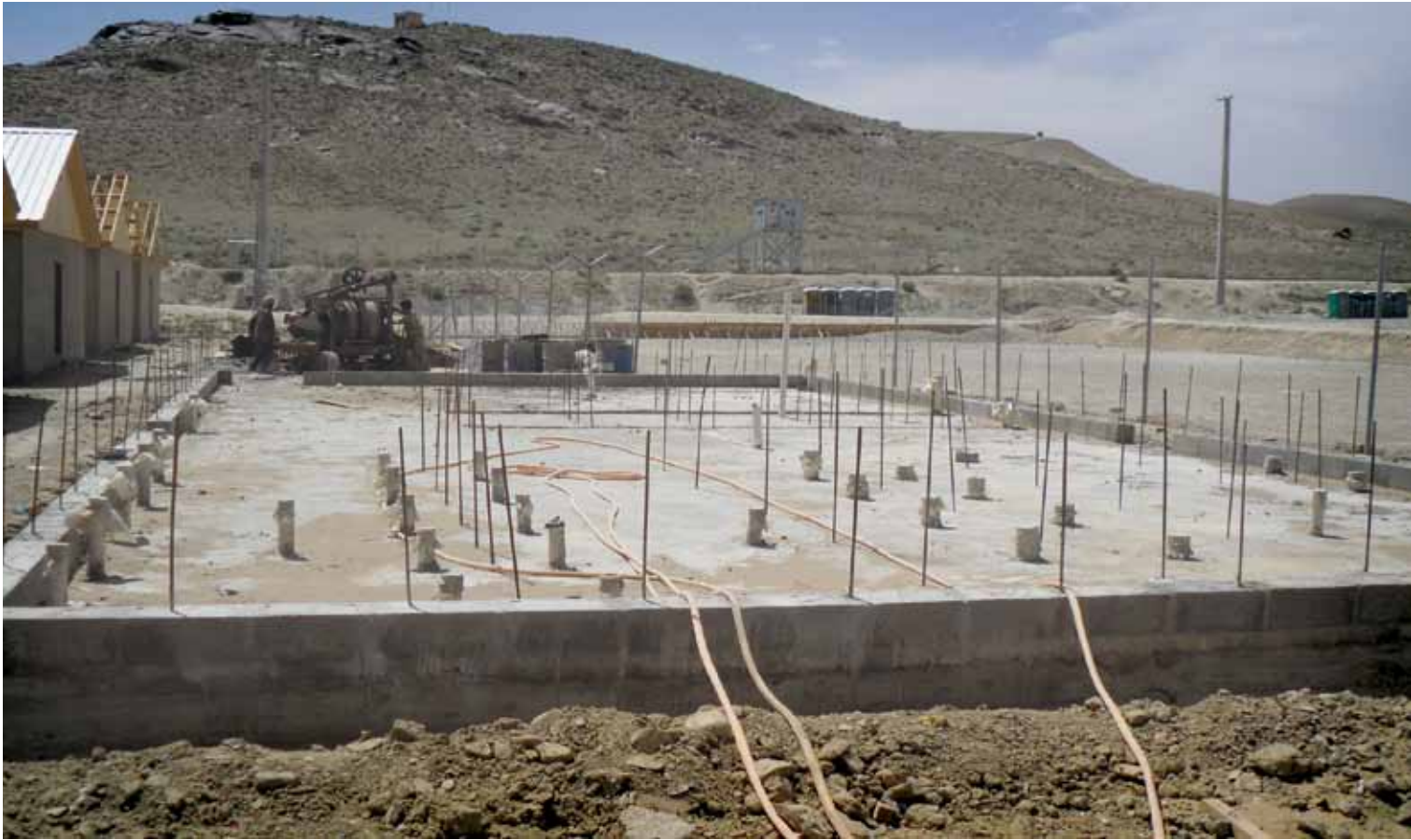
The foundation for a b-hut under construction at Kabul Military Training Center.
