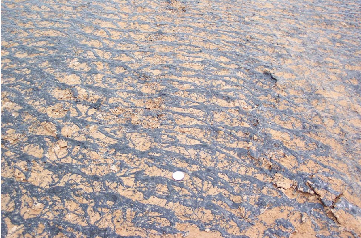
Figure 37. Photo. Results of applying prime at too high viscosity.
