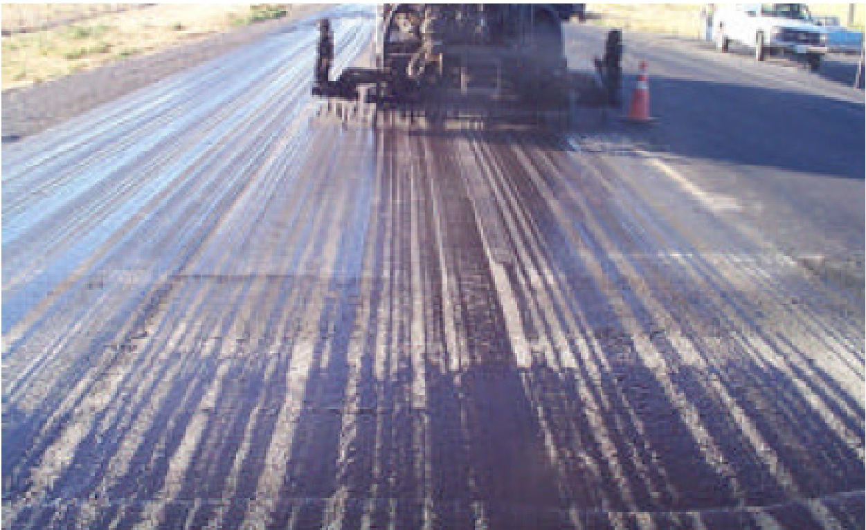
Figure 5. Photo. Non uniform coverage resulting from incorrect spray bar height and/or pump pressure.
