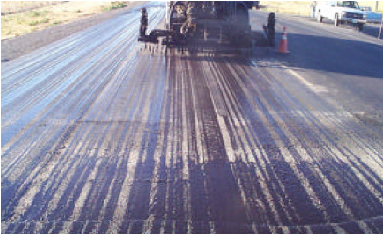
Figure 38. Photo. Streaking in tack coat caused by improper spray bar height and/or pump pressure.
