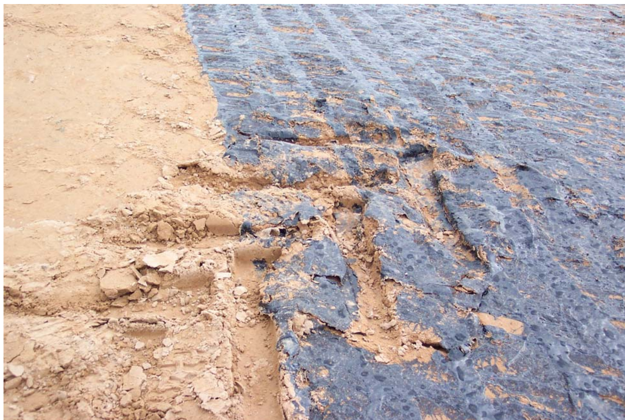
Figure 1. Photo. Lack of penetration of emulsified asphalt prime on silty clay subgrade.
