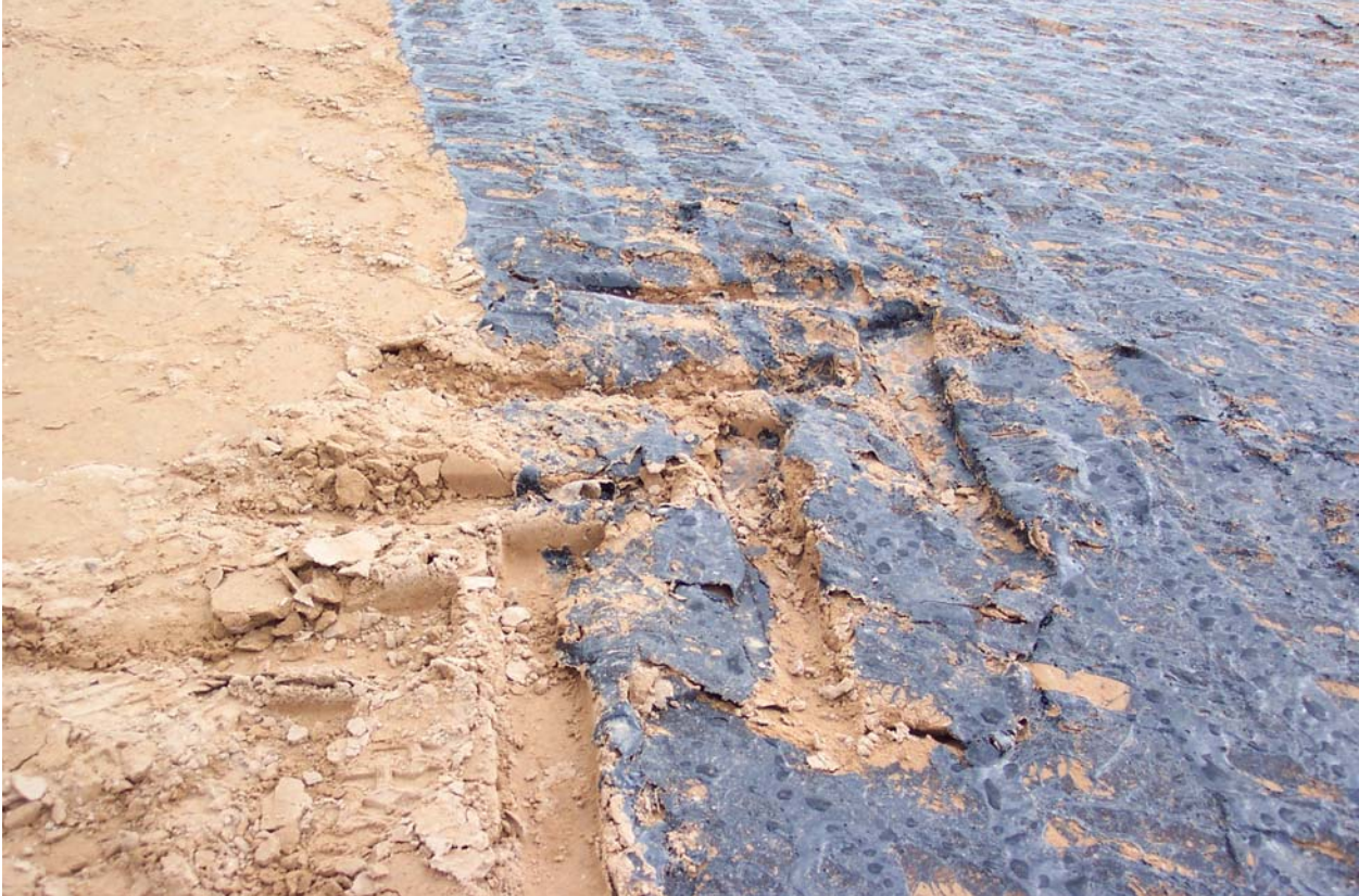
Figure 36. Photo. Poor penetration of prime caused by the high fines content of the base.
