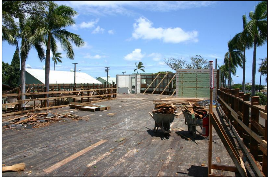
Photo4.HHFaward.BldgRehab: A team of U.S. Army Garrison-Hawaii’s Cultural Resources staff; the U.S. Army Corps of Engineers, Honolulu District; and small business contractor Alutiq-Mele, LLC tackled years of termite damage to rehabilitate and renovate historic Building 330 on Fort Shafter. The building was originally built as the headquarters for the Hawaiian Ordnance Depot and was uniquely designed, balancing modernism and old Hawaiiana architectural styles.
