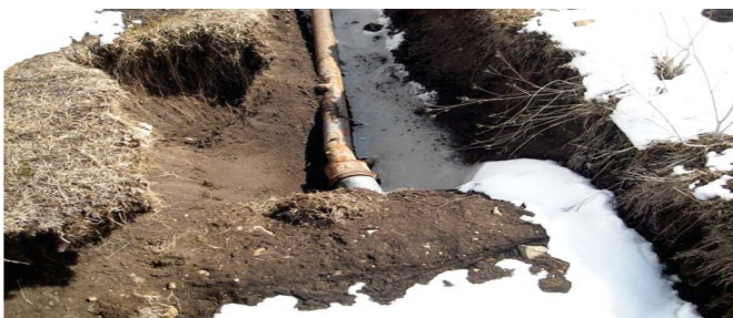
Old damaged pipe led to 30 to 40% loss of water supply to the villages.
