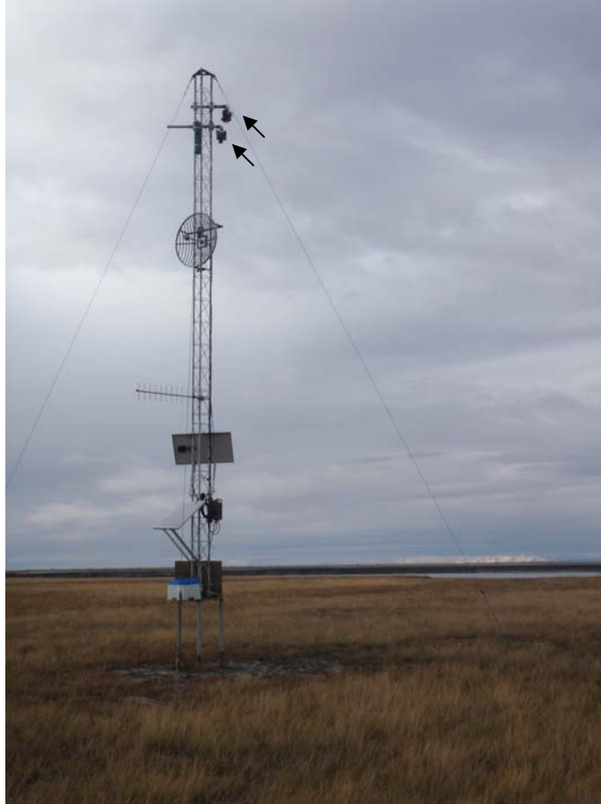
Figure 3: Camera tower with two cameras mounted near the top, arrows pointing towards cameras.
