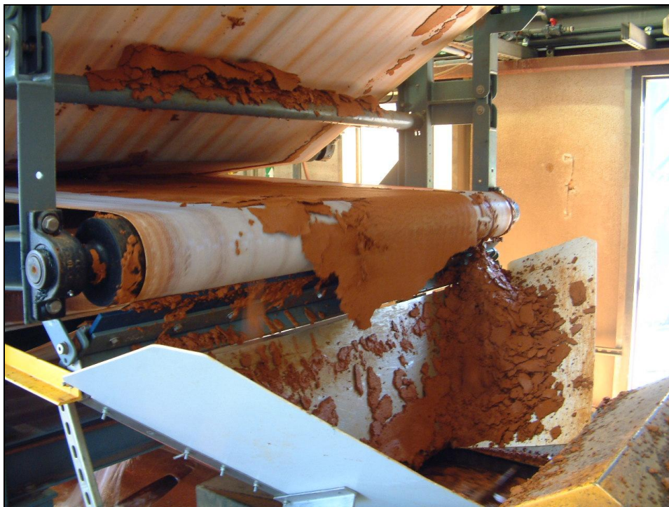
Figure 29. Iron hydroxide peeling off the filter press at the Brandy Camp treatment plant.
