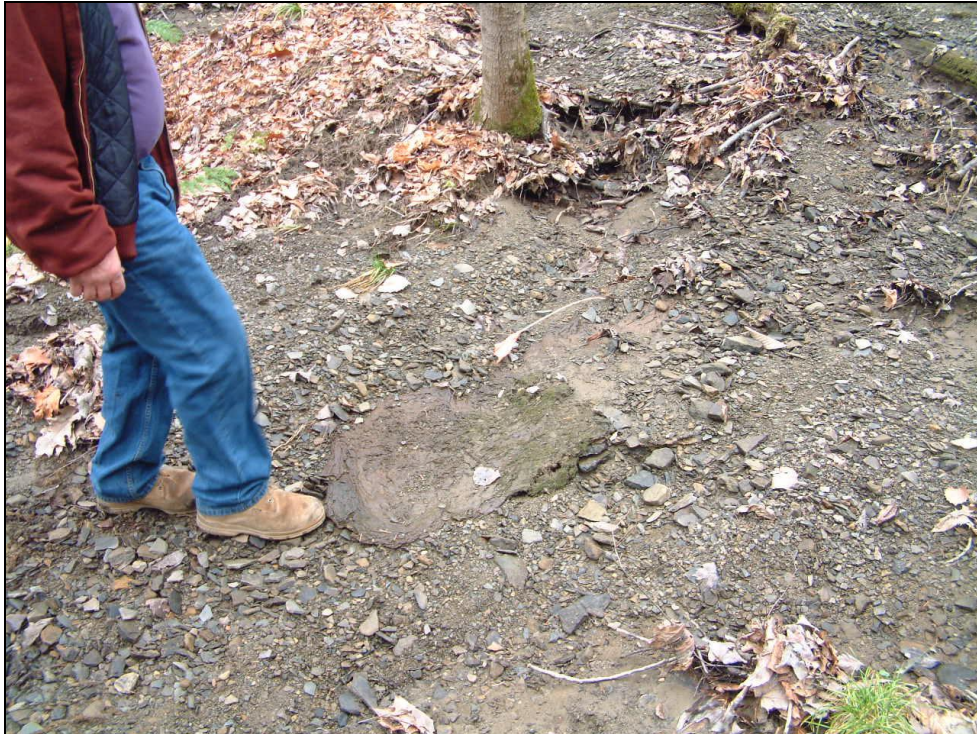
Figure 17. Polyurethane grout exposed in the stream bed in November 2006.
