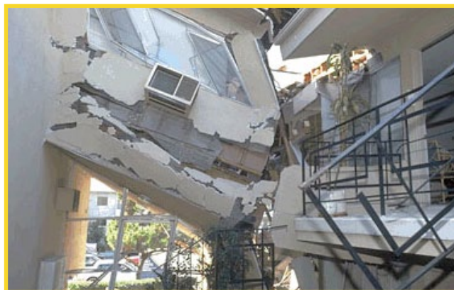
Building damage after an earthquake. Photo courtesy of the USGS.
