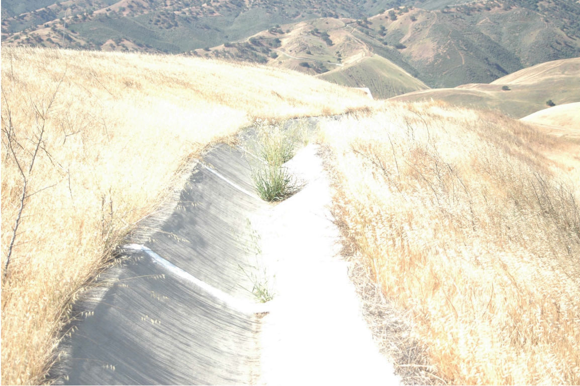
Figure 7 Building 829 Vegetative Growth in Concrete Drainage Ditch
