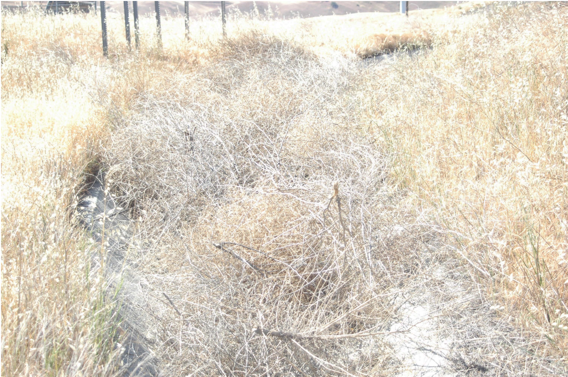
Figure 6 Building 829 Vegetative Debris in Concrete Drainage Ditch
