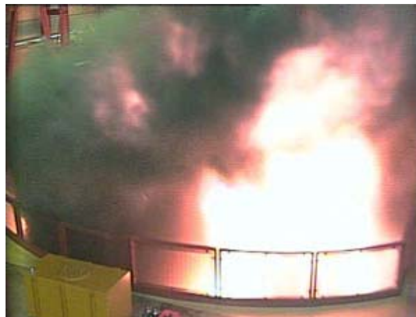
Generator Fire – July 2009
