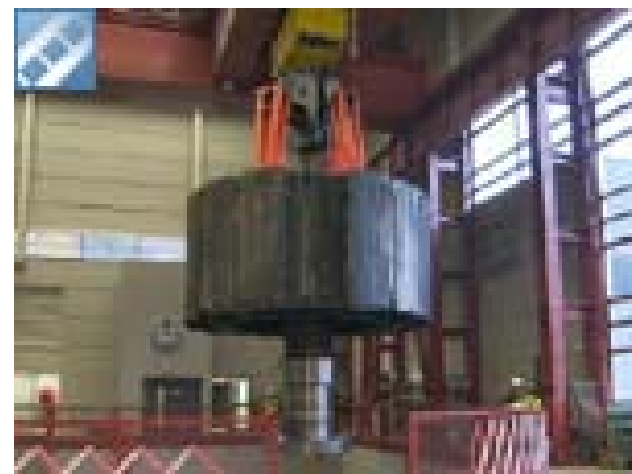
Rotor Removal – December 2009
