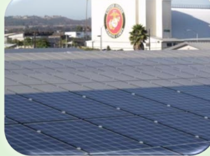
PV System MCAS Miramar
