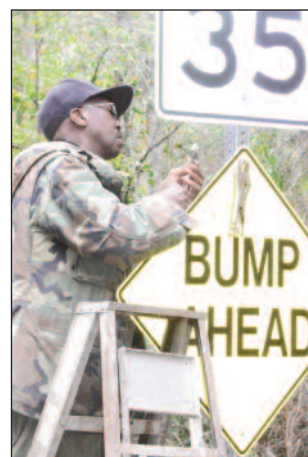
Ronald King, 78th Civil Engineer Squadron Horizontal Shop, removes a caution sign which will no longer be needed following the construction.
