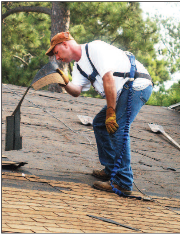
Left, Lee Galpin, a local contractor, removes old shingles from the roof of Friendship pavilion. The other two smaller pavilions require less work which will be completed later this fall.
