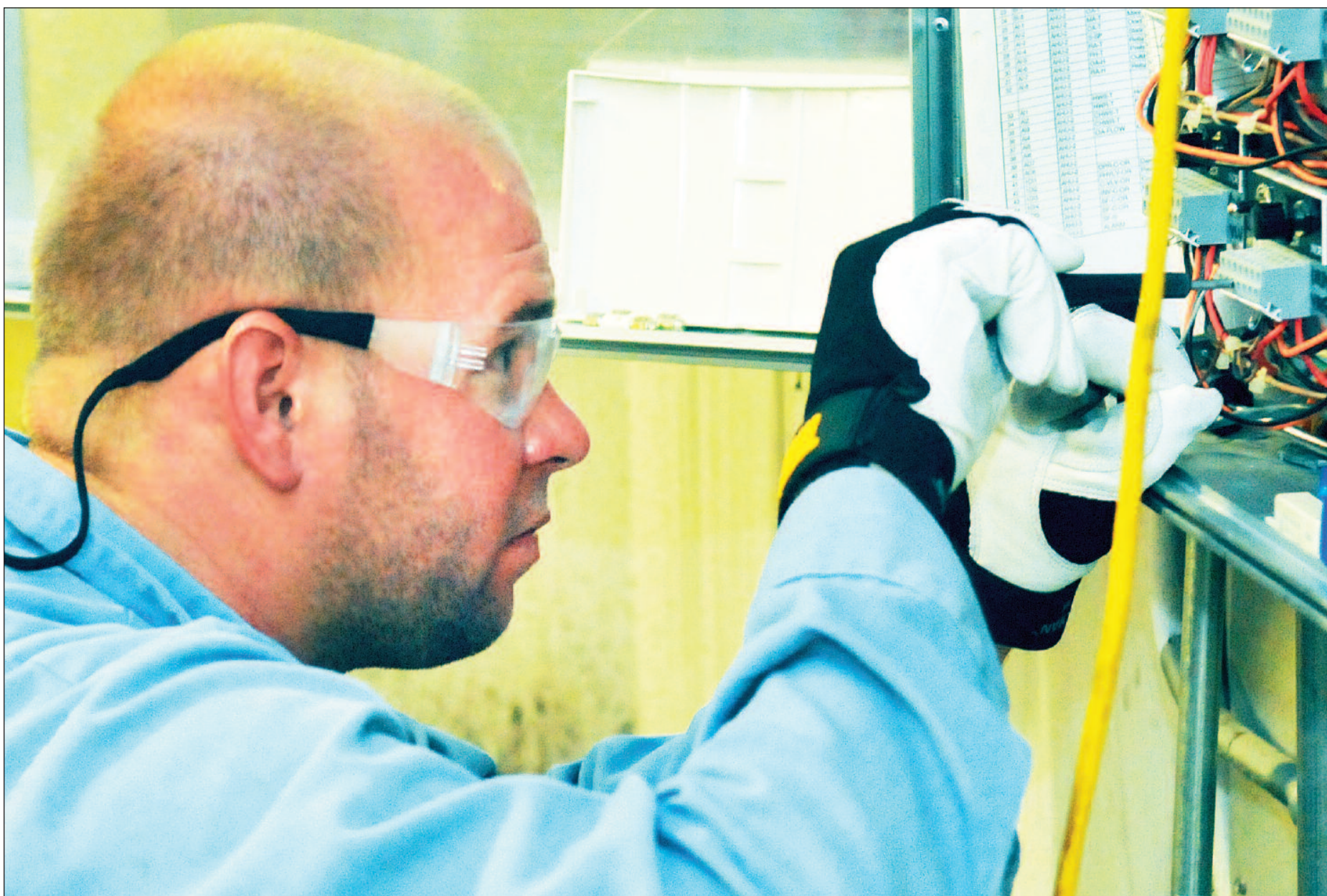
Eric Smith, 78th Civil Engineer Squadron HVAC shop, works on the control panel at the Fitness Center.
