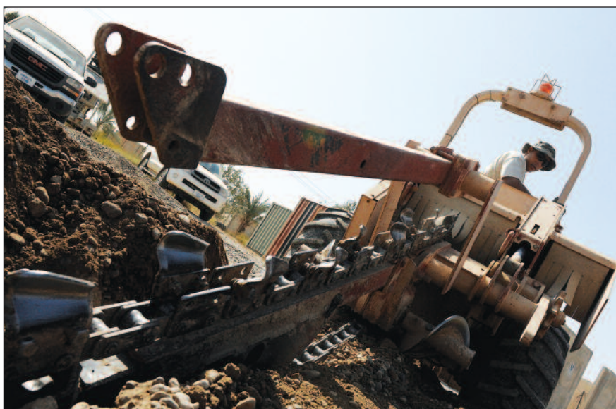
Tech. Sgt. Turvon Casey, 5th Combat Communications Group, operates a trencher to help with the installation of the grounding rods for a tactical communications satellite terminal.
