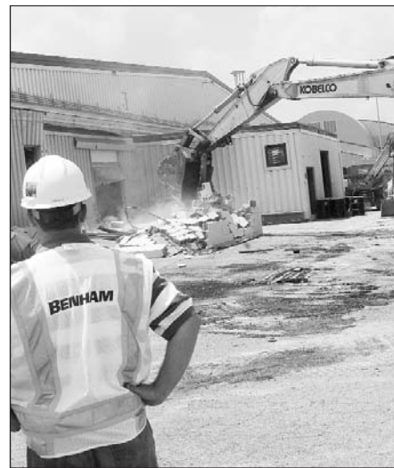
U.S. Air Force photo by SUE SAPP The demolition of Bldg. 148 is part of a construction project which will result in the Advanced Metal Finishing Facility.
