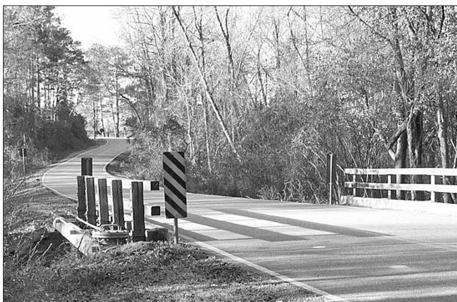
The closure of Hannah Road will allow this bridge to be replaced.
