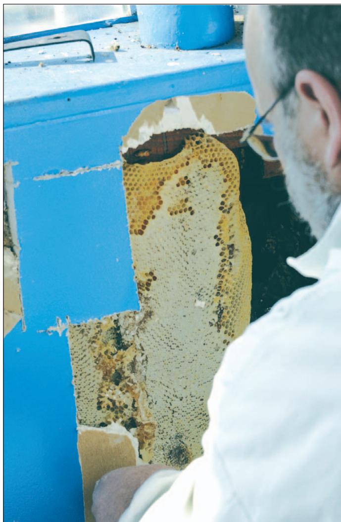
Steve Nofs cuts and removes wall board to expose the bee's honeycomb.
