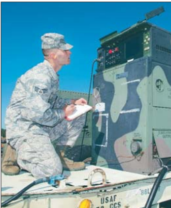
Senior Airman Shaun McVey, 53rd CBCS, performs a two-hour check on a generator used to keep power going during the exercise.
