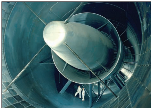
The enormous size of the supersonic circuit compressor of the PWT facility is illustrated by the comparison of workmen standing below the 18-stage compressor. The supersonic circuit is designed to operate at speeds between Mach 1.5 and 4.5 with altitude simulation capability up to 200,000 feet. The compressor – 18 stages in all – is made up of four barrels, three of four stages each, and one of six stages. They can be operated as a unit or one at a time depending on the test conditions. Steel boxes on the walls contain fiberglass pillows for insulation to retain heat when temperature is a test condition.
