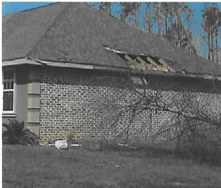
Figure 4.33 Roof Failure on House
