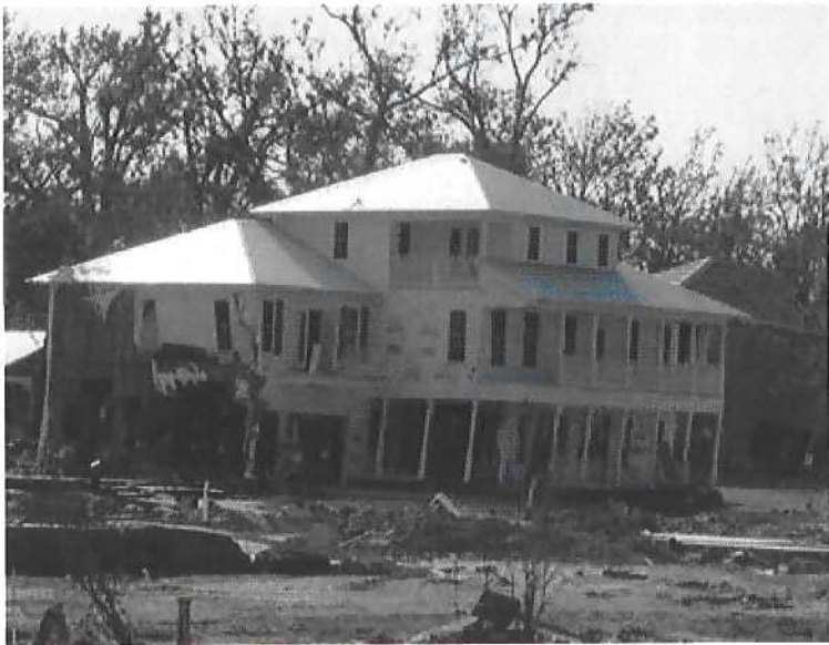
Figure 4.36 Side-Sway Failure in Wood House
