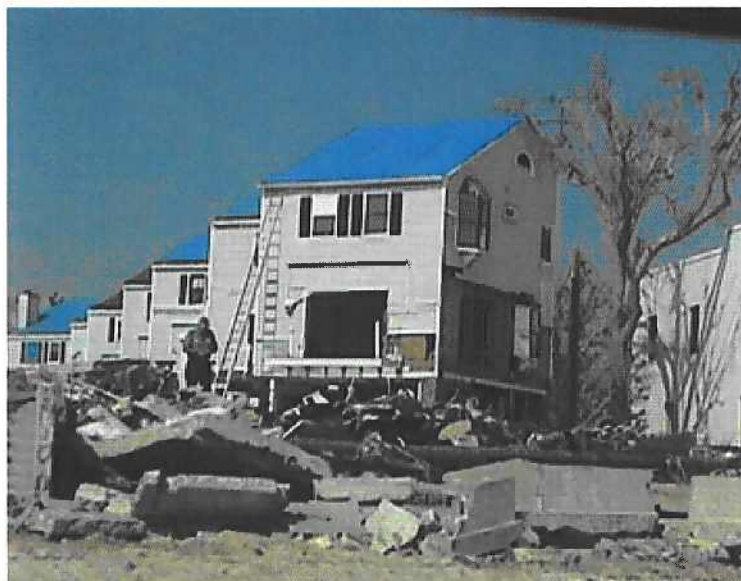
Figure 4.35 Siding Damage on Wood Building
