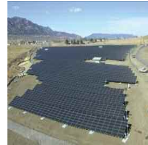
The largest solar power site in the Army, constructed on a closed landfill, will soon supply power to Fort Carson, Colo
