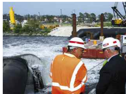
Former Secretary of the Army Dr. Francis J. Harvey is briefed by U.S. Army Corps of Engineers officials at the 17th Street Outfall Canal and Pumping Station in New Orleans Oct. 2, 2006. Harvey toured flood-ravaged New Orleans and USACE's efforts to repair the damaged facilities. Photo by: Betsy Weiner. Date: October 5, 2006. Courtesy of US Army from: http://www4.army.mil/OCPA/uploads/large/2006/OCPA-2006-10-05-131652.jpg .
