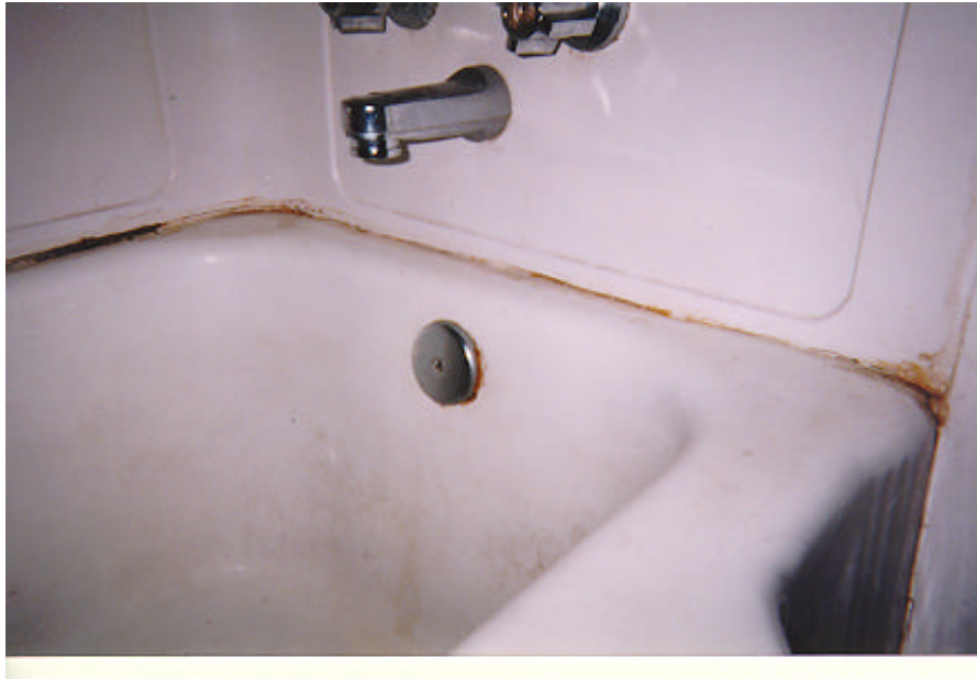
Bathtub surround improperly installed, Avenal, CA
