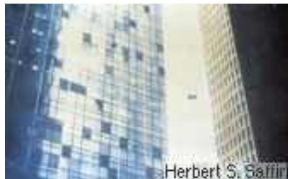
Windows falling from a high-rise building
