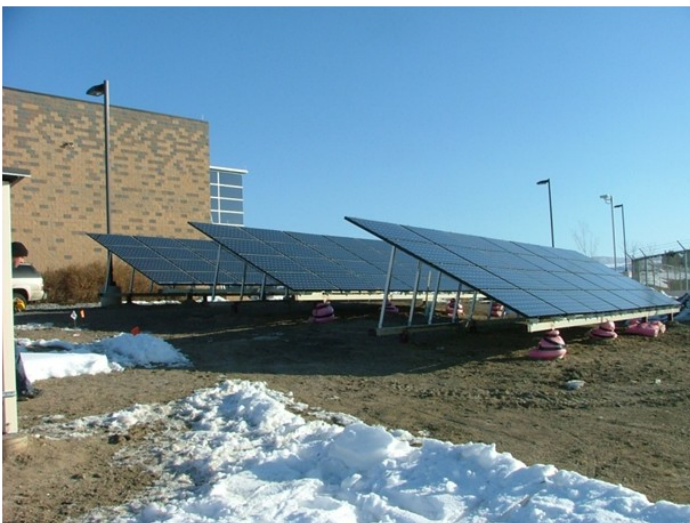
New photovoltaic system at Grand Junction Air Center
