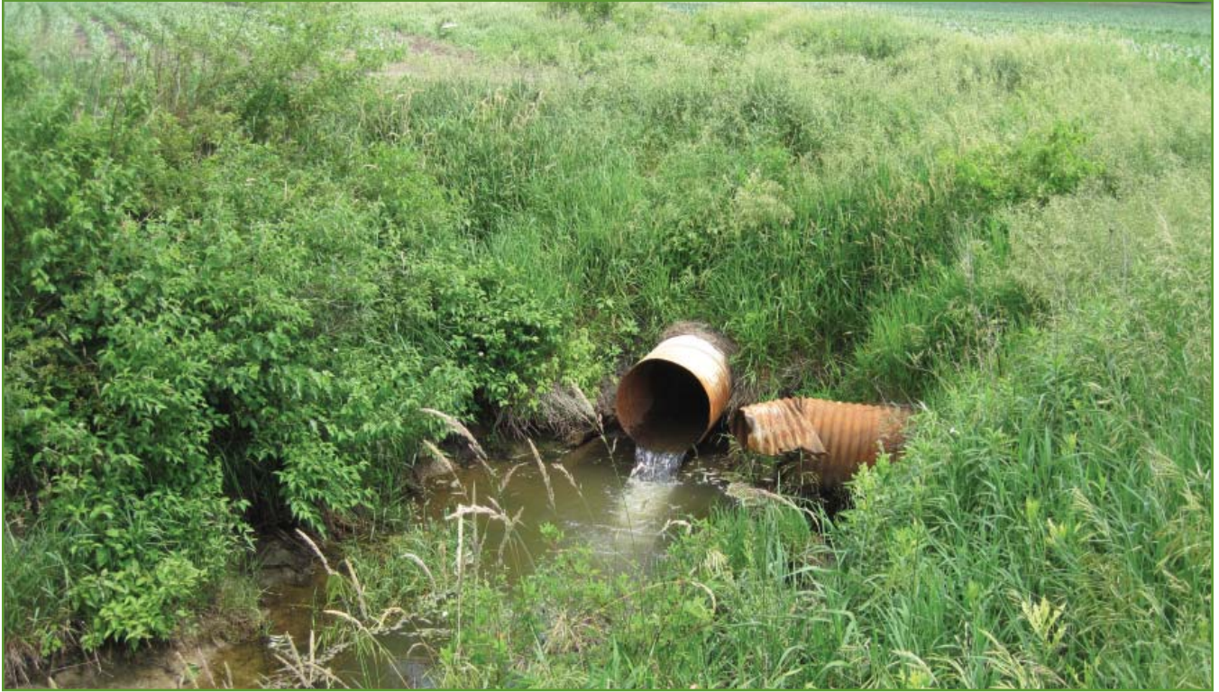
Figure 11: Water flowing into Parker-Cobb Ditch through 27-inch (69 cm) CMP from West Fork Parker Ditch. Photo by USACE.
