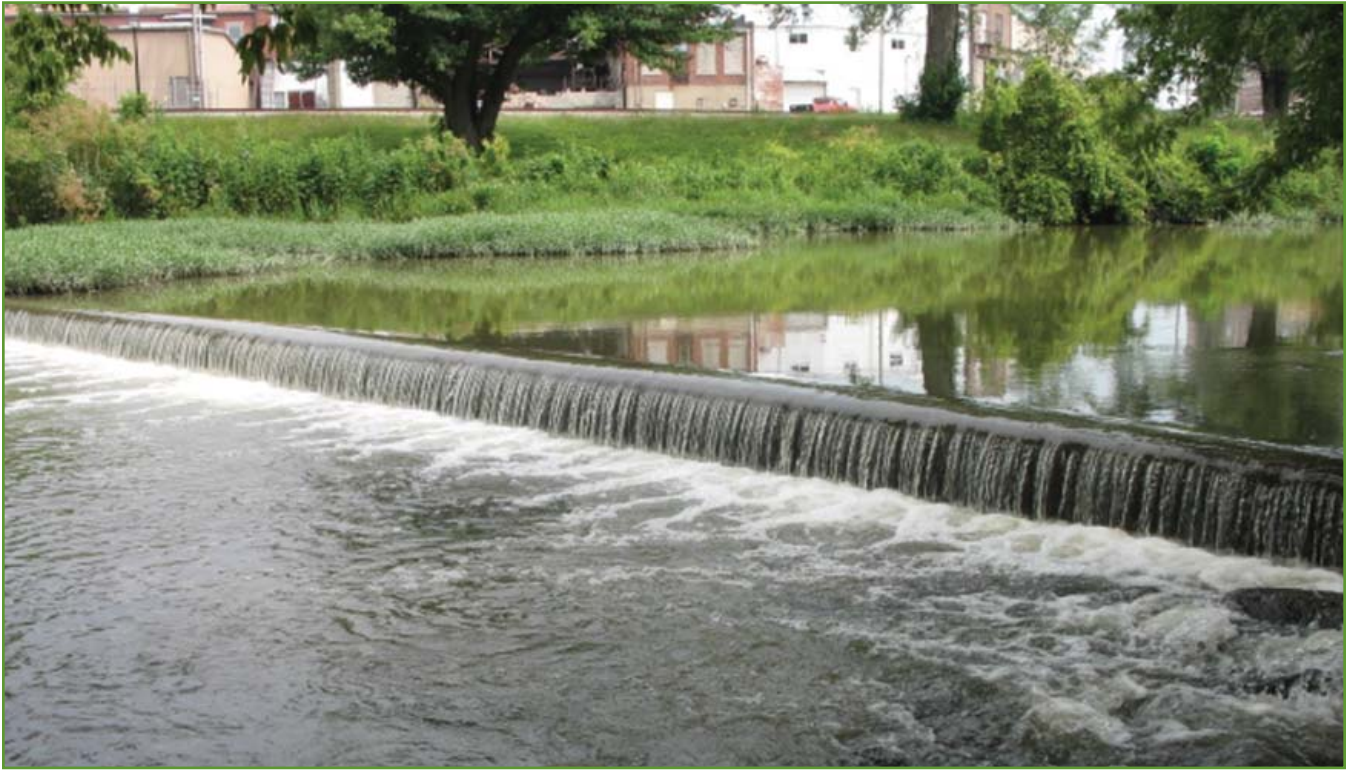
Figure 27. Small low head dam on the Little River downstream of S. Jefferson St. Bridge. Photo by USACE.
